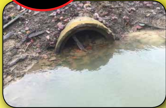
Improper drainage = poor track structure
